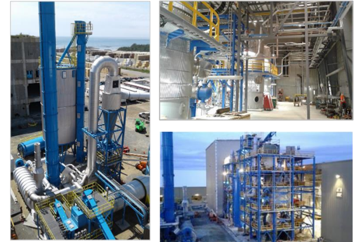
Cote Nord, Quebec, 10M gpy commissioned 2018
