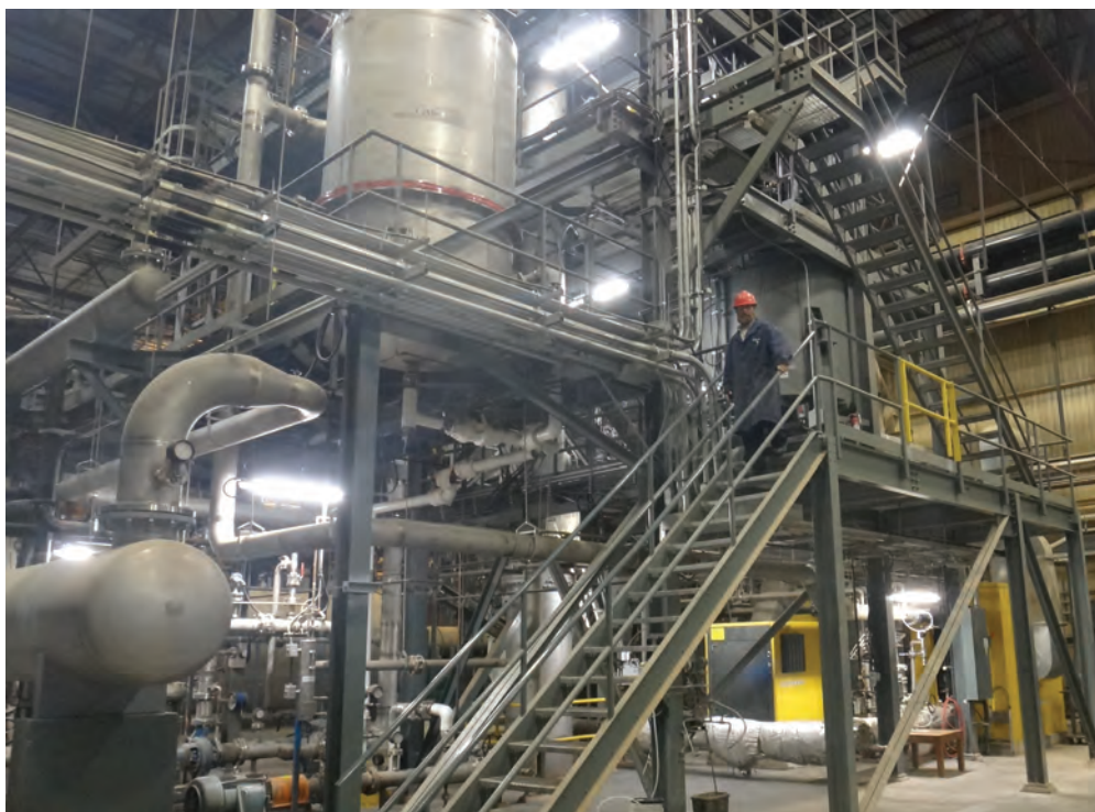
Ensyn's pyrolysis facility.
